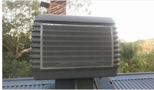
Evaporative cooler ember guards
