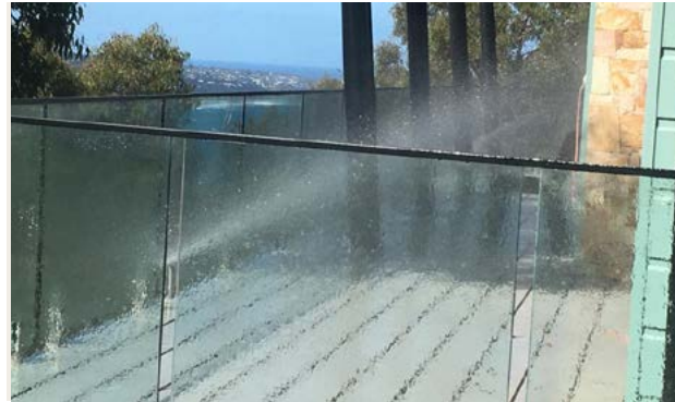
Sprinkler nozzles targeting deck and windows
