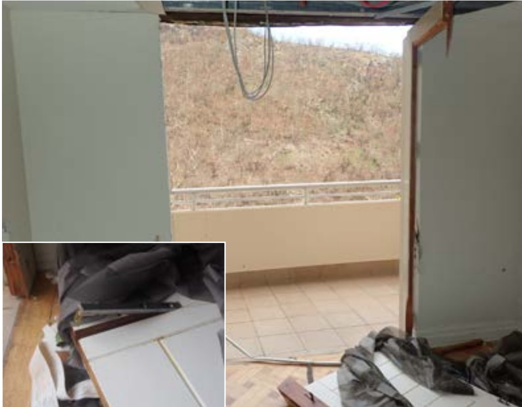
A door that had inadequate fixing to the wall frame and inadequate door latches
