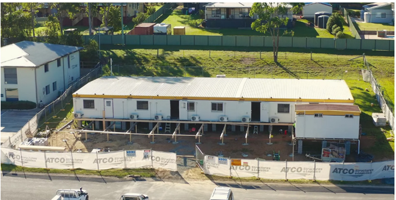
Construction of the Mogo pop-up mall with donated demountables. Credit: Business Council of Australia.
